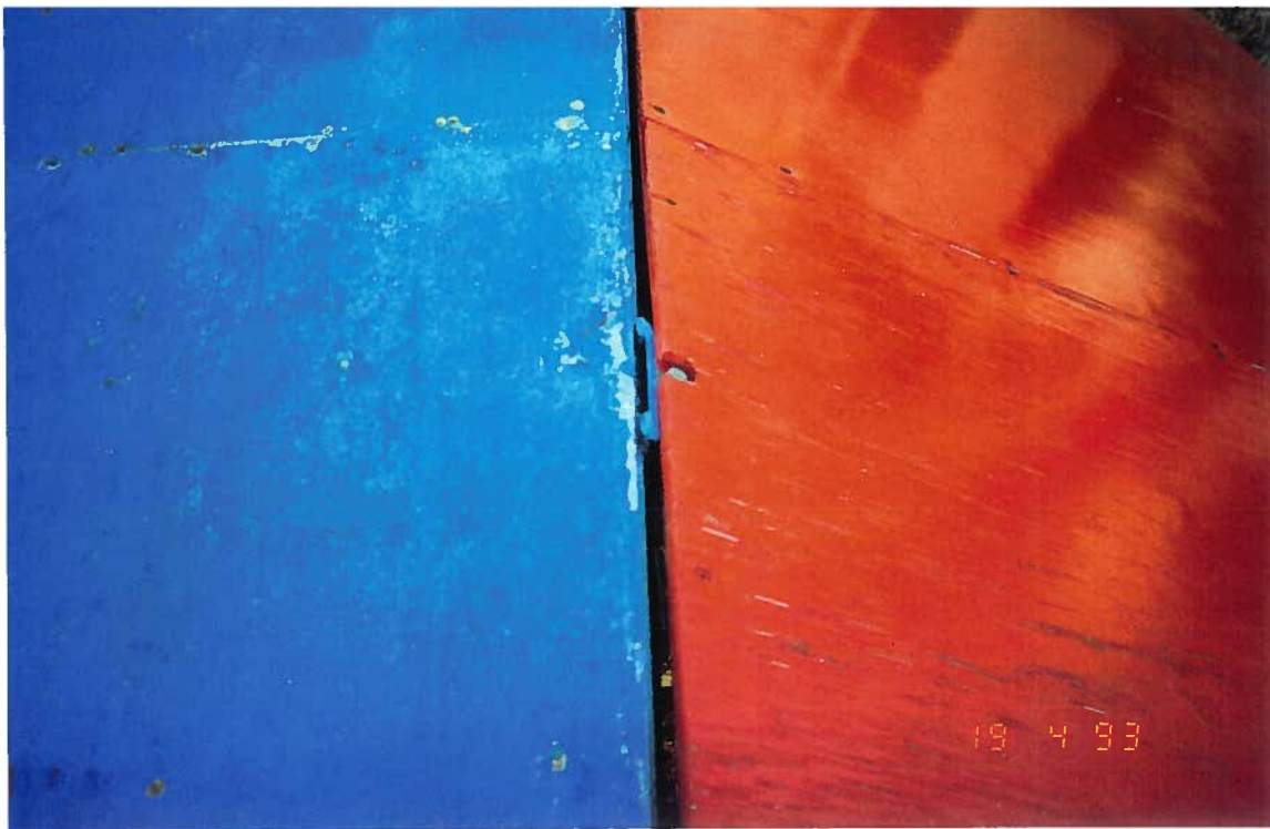
WING BOLTED TO THE DECK FRAME. NOTE THAT THE BOLT HEAD IS RECESSED.
