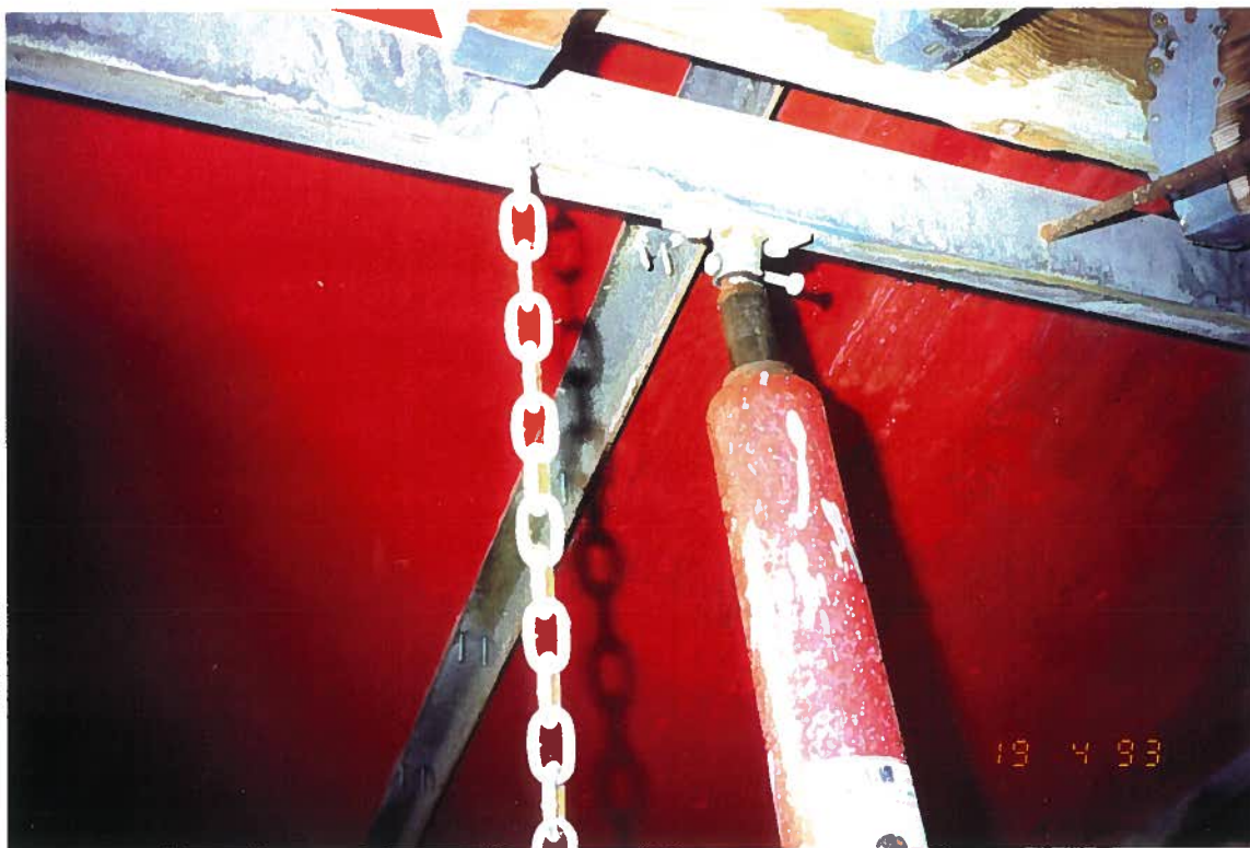
TOP OF JACK BOLTED INTO NIPPLE. NOTE THE TIE ROD DRILLED THROUGH THE DECK TRISS.
